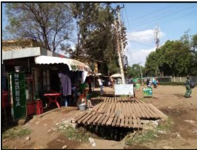
Figure 5. Example of a Fabricated Wooden Drainage Cover
