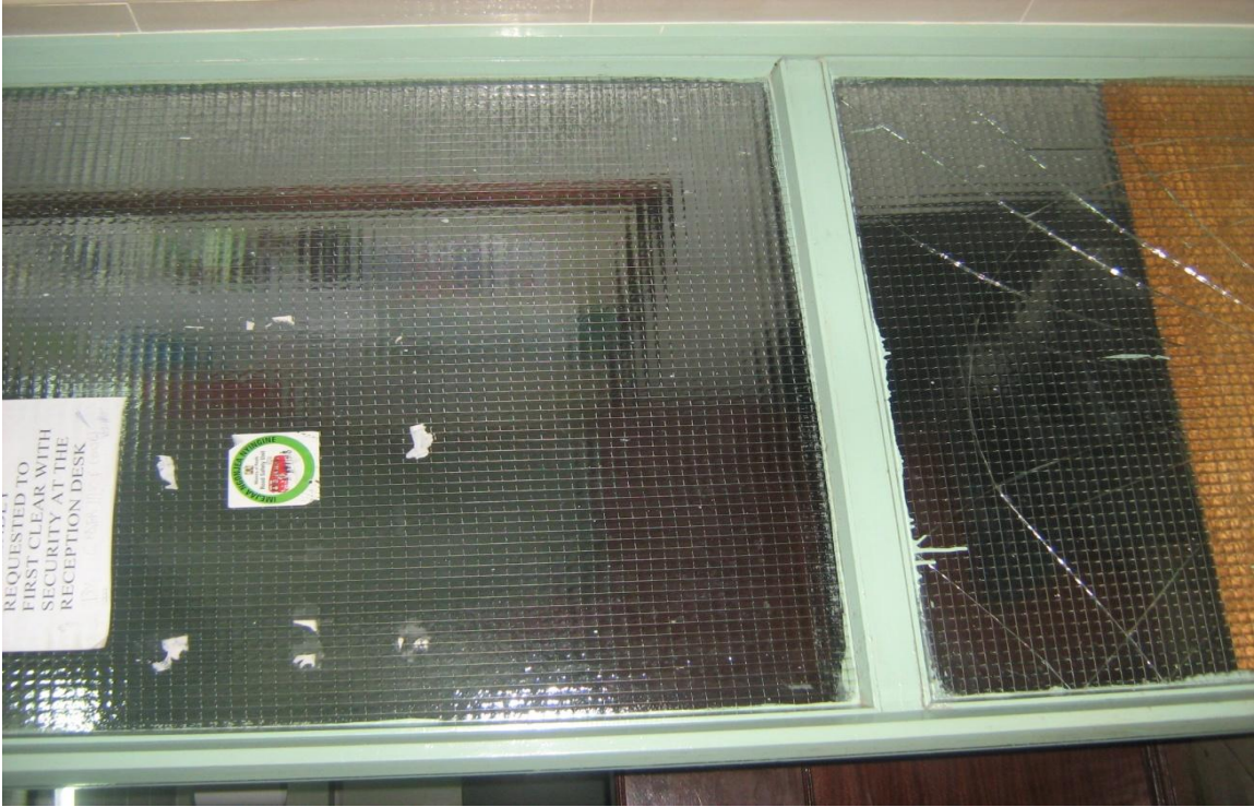
Photograph A17: Window with Cracked Glass Pane at Transcom House. The glass pane breakage may be as a result of the users being negligent.
