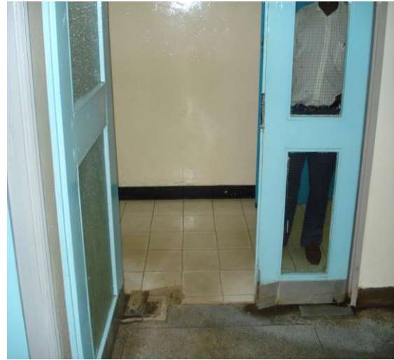
Photograph 4.2: Double Door with Loose Hinges at the Magereza House Attributed to Negligence. The defect requires negligible effort to repair.
