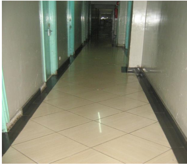
Photograph 4. 20: Recently Laid Porcelain Tiles Floor Finish to Transom House as a Major Maintenance Work.
