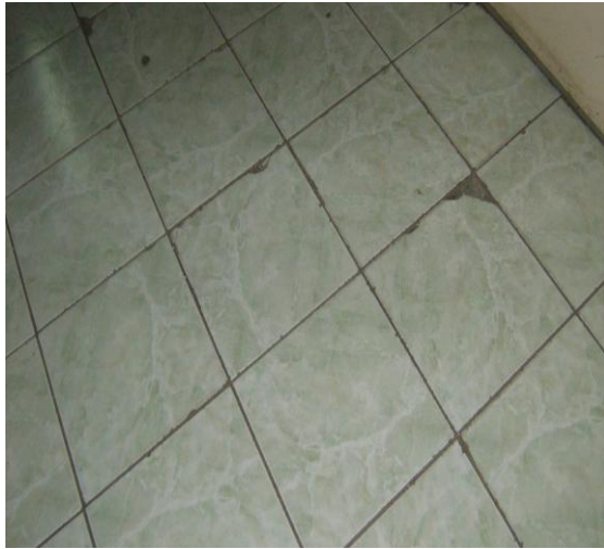
Photograph 4.11: Defective Ceramic Floor Finish at Sheria House Attributed to In-appropriate Specification.
