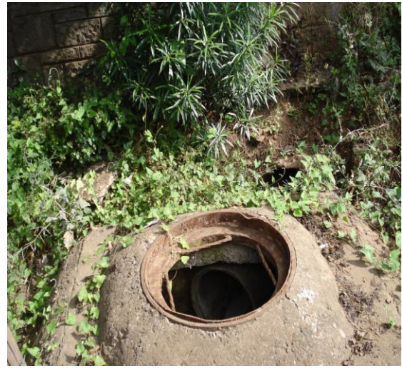
Photograph 4.10: Missing Manhole Cover at NSSF Building Attributed to Vandalism.
