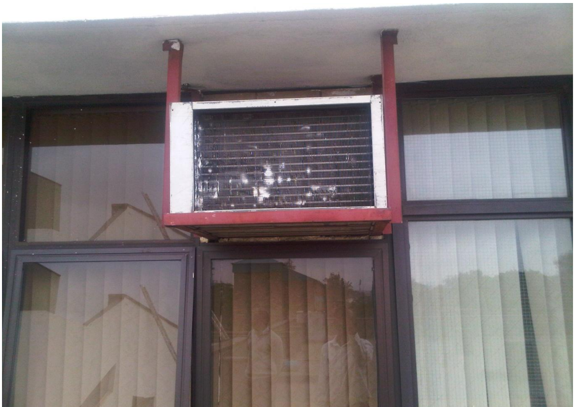
Photograph A8: Window with Broken Glass Panes at National Cereals and Produce Board Building.
