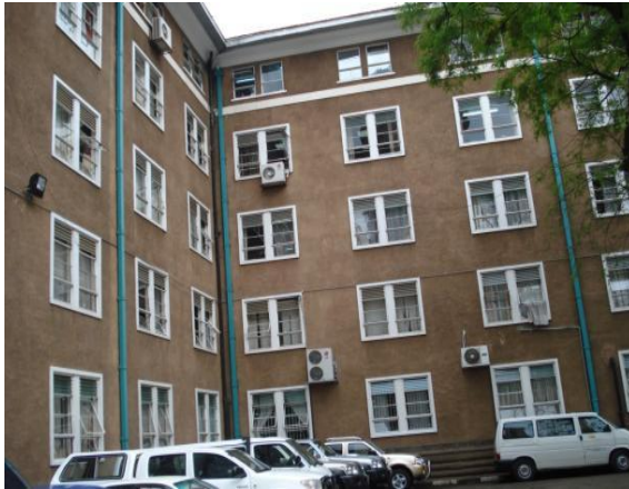
Photograph 4. 38: Tyrolene Finished External Façade of Jogoo House A, a Cost Effective Finish .Jogoo House A is finished in tyrolene finish which although dull provides a cost effective maintenance solution.
