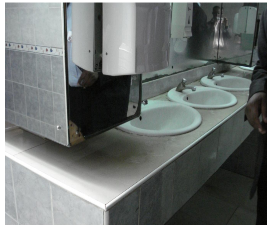
Photograph 4. 17: Newly overhauled Plumbing/ Drainage in Washrooms to Kenyatta International Conference Centre Building as a Major Maintenance Work.
