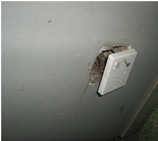
Photograph 4.3: Loose Electrical Power Socket at Works House Attributed to Careless Movement of Furniture or Goods. This requires negligible effort to repair.
