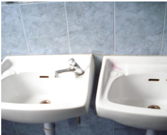
Photograph 4. 40:Use of Ceramic Tiles to Washrooms to Jogoo House A, a Cost Effective Internal Cladding Material. Ceramic tiles are water proof and therefore suitable in wet areas like washrooms and Kitchenettes. Cost in use is very low but higher initial cost than paint.
