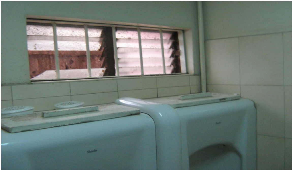
Photograph A4: Kitchenette Window of Public Service Commission Building with Missing Louvre Glass Blades.
