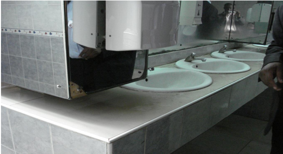
Photograph A3: Use of Ceramic Tiles to Washrooms to Kenyatta International Conference Centre Building
