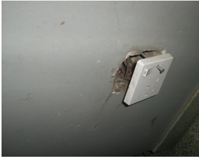
Photograph 4. 24: Re-Screwing of Loose Electrical Power Socket and Damaged Power Switch at Works House as a Minor Maintenance.
