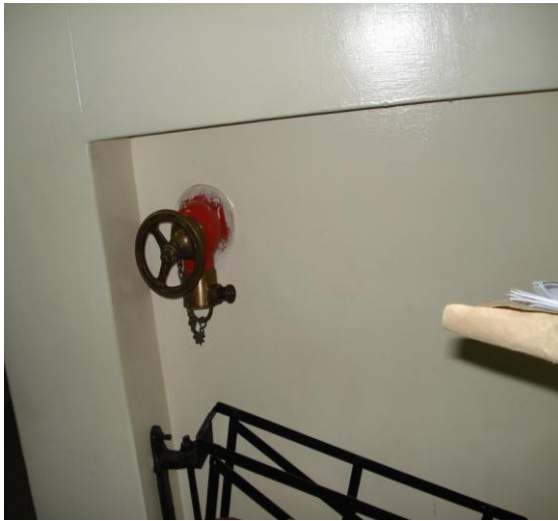
Photograph 4.9: Missing Firefighting Hosereel Equipment at Jogoo House A Attributed to Vandalism.
