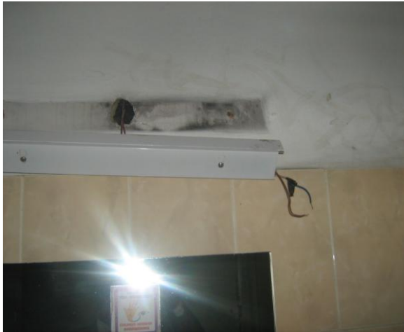
Photograph 4.5: Loosely Hanging Fluorescent Lighting Fittings at Transcom House Attributed to Negligence.
