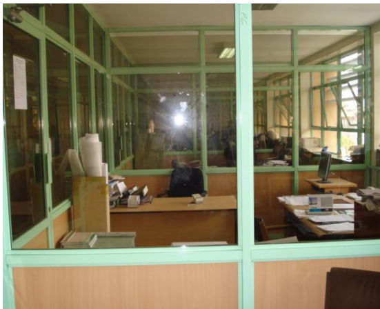
Photograph 4. 16: Newly Overhauled Partitions to the 7 th Floor, Works Building Leading to Overhaul of Electrical Installation Work as a Major Maintenance Work.
