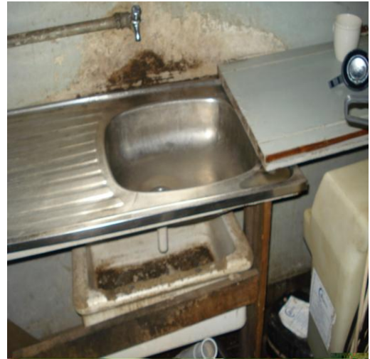
Photograph 4.12: Damaged Kitchenette Timber Work Top and Peeling Paint Due to Dampness at Jogoo House A Attributed to Deficient Design.
