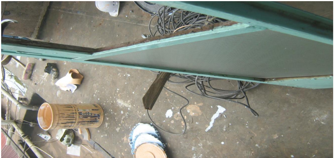
Photograph A6: Missing Glass Pane to the Access Door to Machine Room of Works House This may be as a result of hard bangs by users.
