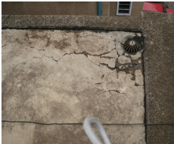
Photograph 4.13: Failed KICC Flat Roof Attributed to In-ability to Regularly Replace the Water Proofing Membrane Due to Budgetary Constraints.
