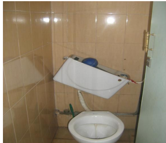
Photograph 4.4: Loosely Hanging Flush water Cistern at Transcom House attributed to Negligence This requires negligible effort to repair.
