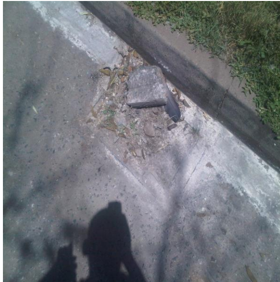
Photograph 4. 19: Failed Parking of National Cereals and Produce Board Parking calling for Re-carpeting as a Major Maintenance Work.
