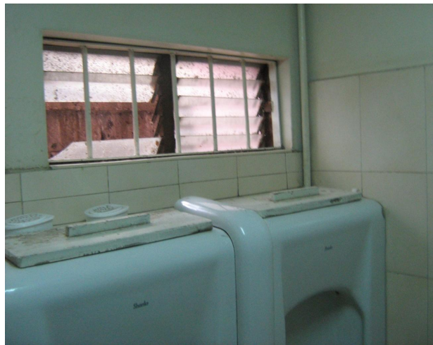
Photograph 4. 21: Replacement of Missing Louvre Glass Blade to Public Service Commission Building as a Minor Maintenance Work.
