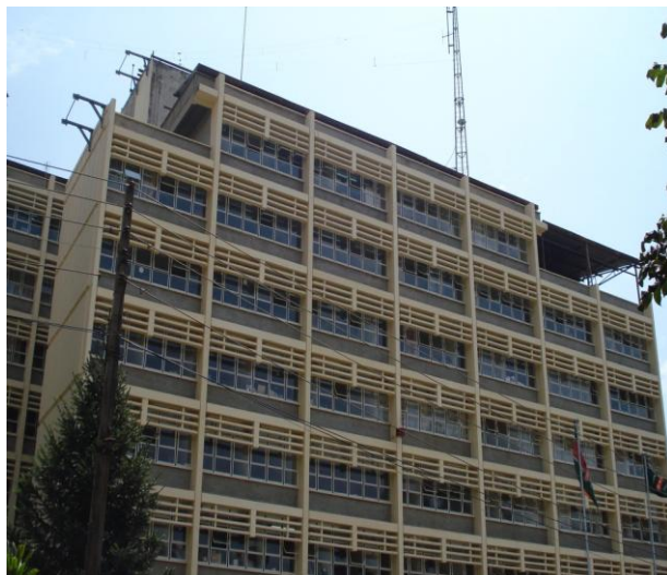
Photograph 4. 14 : The Ongoing Re-Roofing Works to Magereza House as a Major Maintenance Work.
