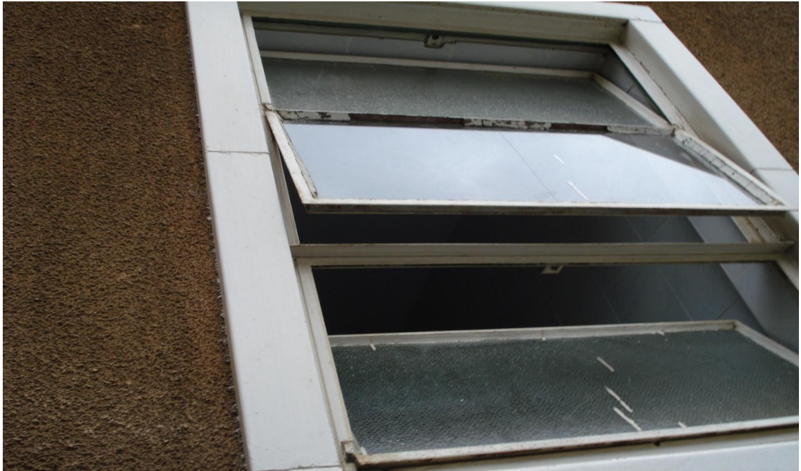
Photograph A5: Window with Fallen Glass Panes at Jogoo House A This is mostly attributed to negligent handling
