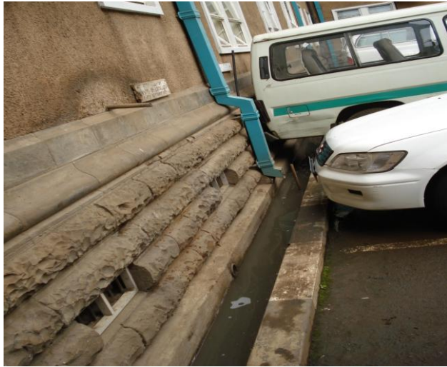
Photograph 4. 25: Clearance of Blocked Storm Water Drainage at Jogoo House as a Minor Maintenance Work.
