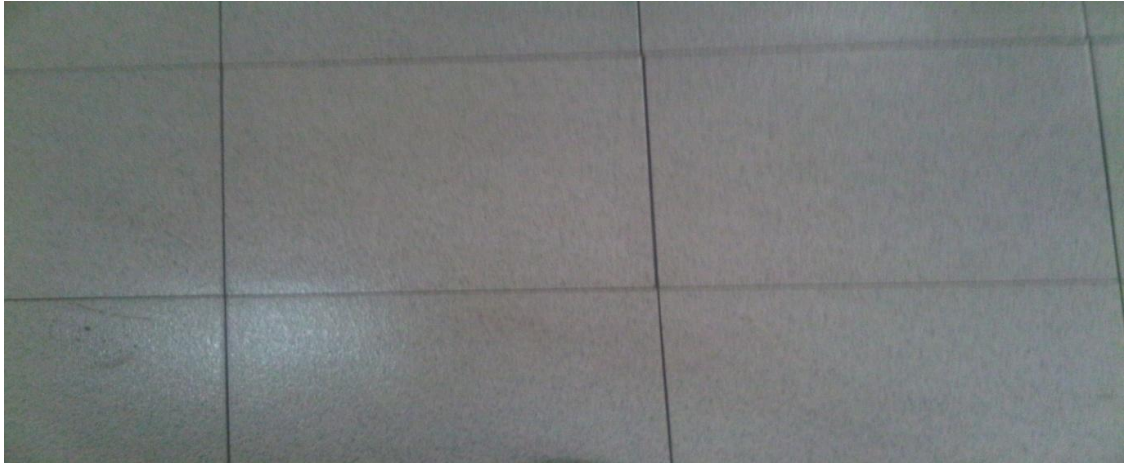
Photograph A1: Floor Finish to Safety House
