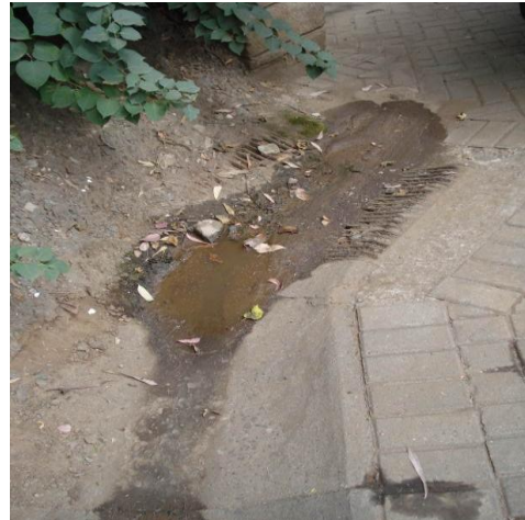
Photograph 4.6: Blocked Storm Water Drainage Gully Pot at Transcom Parking Attributed to Negligence.
