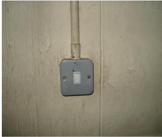
Photograph 4. 18: Old Out-dated Surface Wiring at Jogoo House Calling for Overhaul of Electrical Installation as a Major Maintenance Work.
