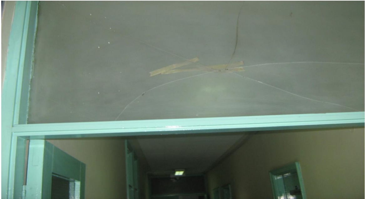
Photograph A7: Door Fan Light with Cracked Glass Pane at Works House. This is attributed to negligent handling
