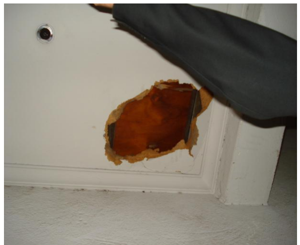
Photograph 4.8: Ceiling Board damaged by Leaking Tiled Roof at Jogoo House Attributed to Poor Supervision. Continued state of affairs might further damage more building components
