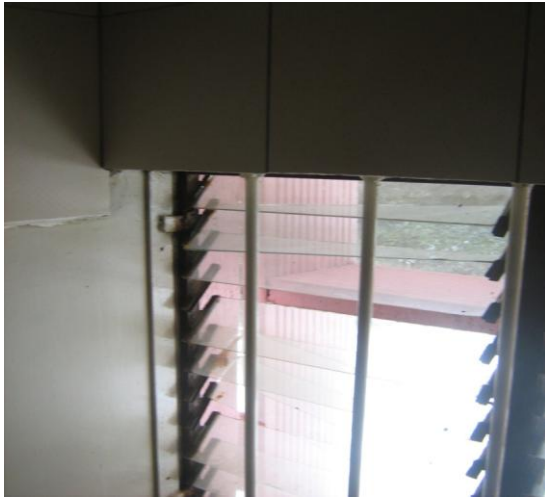
Photograph 4.1: Precariously Hanging Loose Glass Louvres of Public Service Commission Building Attributed to Negligence. The defect requires negligible effort to repair.
