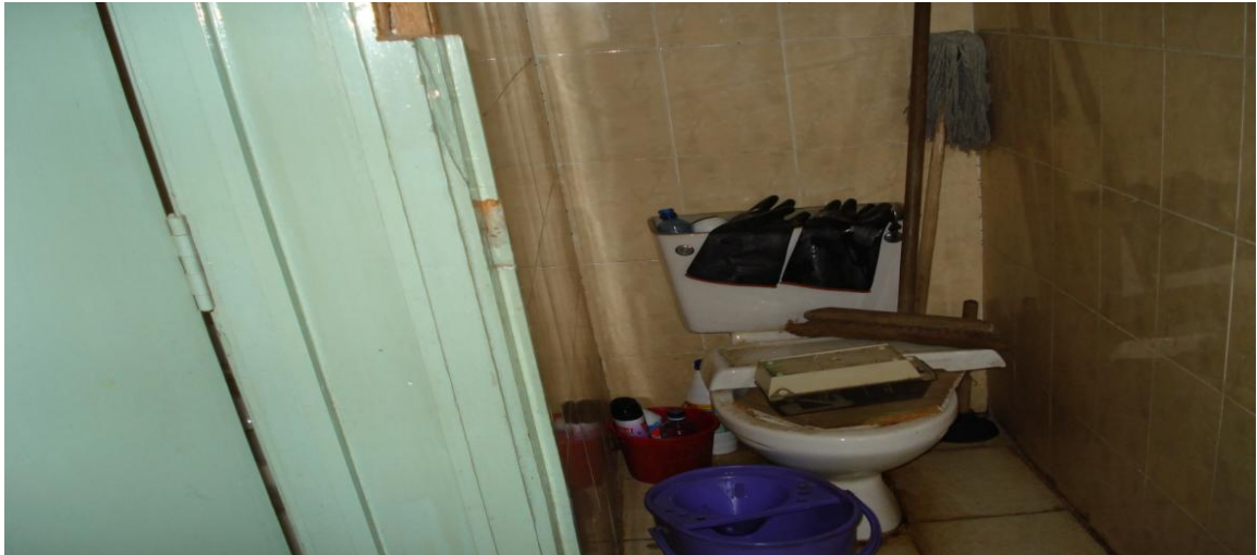
Photograph A15: Broken Down Flush Water Cistern and Water Closet at National Social Security Fund Building
