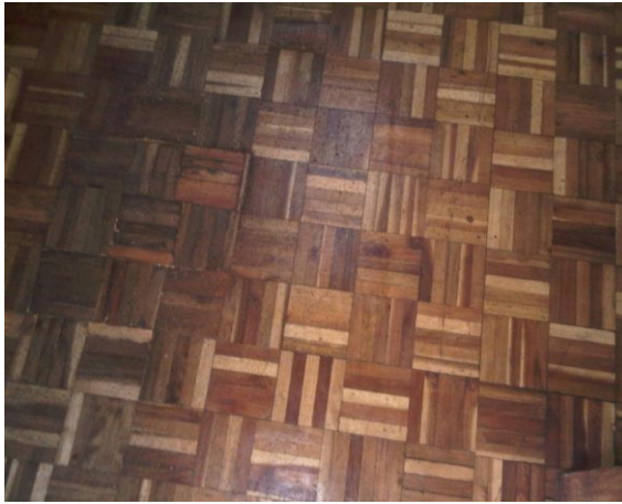
Photograph 4. 26: In-appropriate Choice of Parquet as Floor Finish to NCPB House. Parquet cannot withstand wear and tear subjected from space use impacts.
