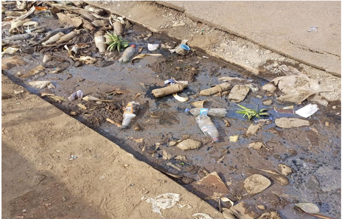
Figure 4. 4: Blocked drainage due to improper garbage disposal. (Daraja Mbili market)
