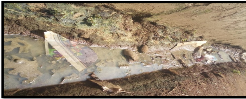
Figure 3: Stagnant Water Due to Poor Drainage in Nyalenda Estate in Kisumu City Source: Survey Data, 2023
